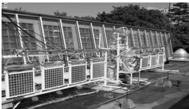
Figure 1: Closed grower systems at the University of Pannonia
