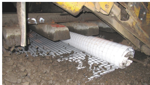
Figure 2: Construction geogrid-reinforced trial railway track on line Lebeny-Mosonszentmiklos (Hungary) on 25 th of May in 2010 with Geogrid type 2
