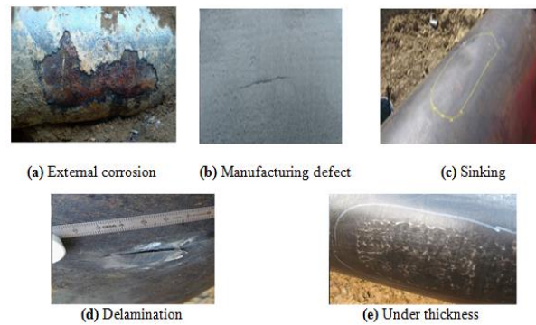
Figure 1: The studied types of pipeline defects
